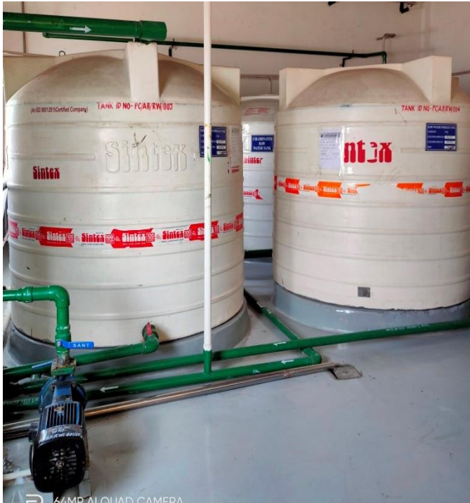
Step 1: Raw water stored in HDPE storage tanks
