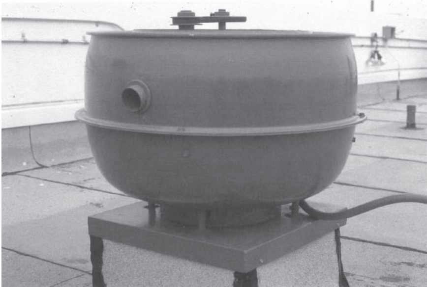
Figure 7-2. Power roof ventilator
