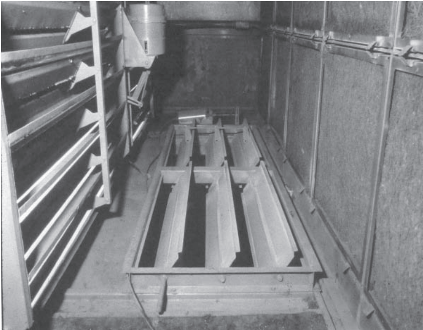
Figure 8-14. Parallel blade dampers in mixed air plenum. Notice blade action for opposed blade and parallel blade dampers.
