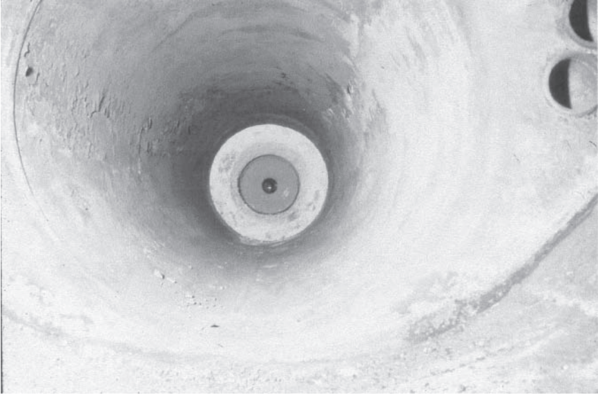
Figure 3-6. Combustion Chamber and Fire Tubes. Two-pass Boiler
