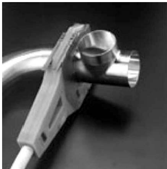
Fig. 4 Automatic orbital welder in the process of joining two long tangent stainless steel fittings.
