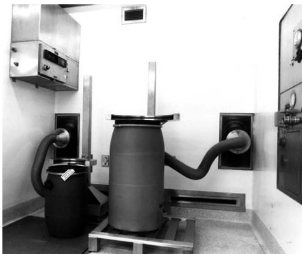
Fig. 8 Weighing and dispensing room. Each mauser drum has special extraction units that fit directly over the variously sized drums.
