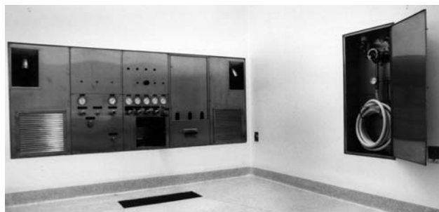
Fig. 4 Multipurpose room with an easily cleanable covered terrazzo floor, dry-wall fiberglass mat with epoxy-painted walls, floor drain, and utility panel. The room has a self-contained hot and cold water wash-down capability.
