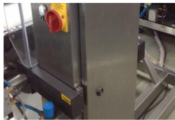
Inside Electric Panel
