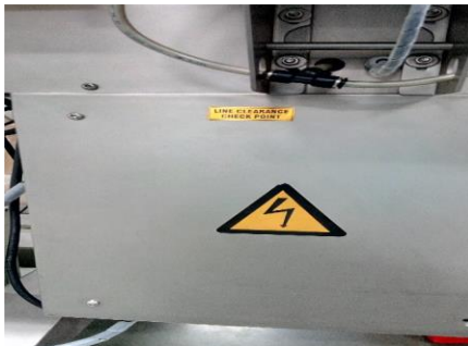
1) Inside the electrical panel
