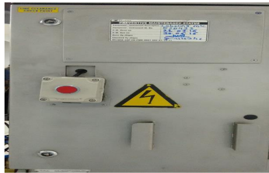
2) Inside the electrical panel.
