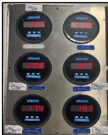
Figure 12: Adjacent areas having Pressure Differential within limit
