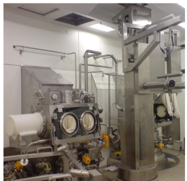
API production facility
